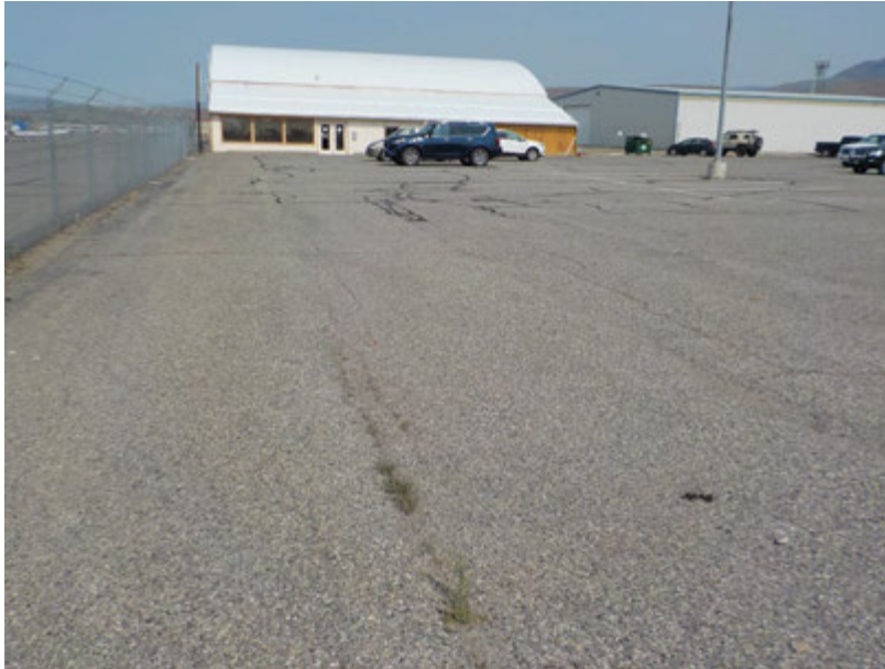
View of parking and southeast side of GA Terminal Building (looking west from east boundary of subject property).
