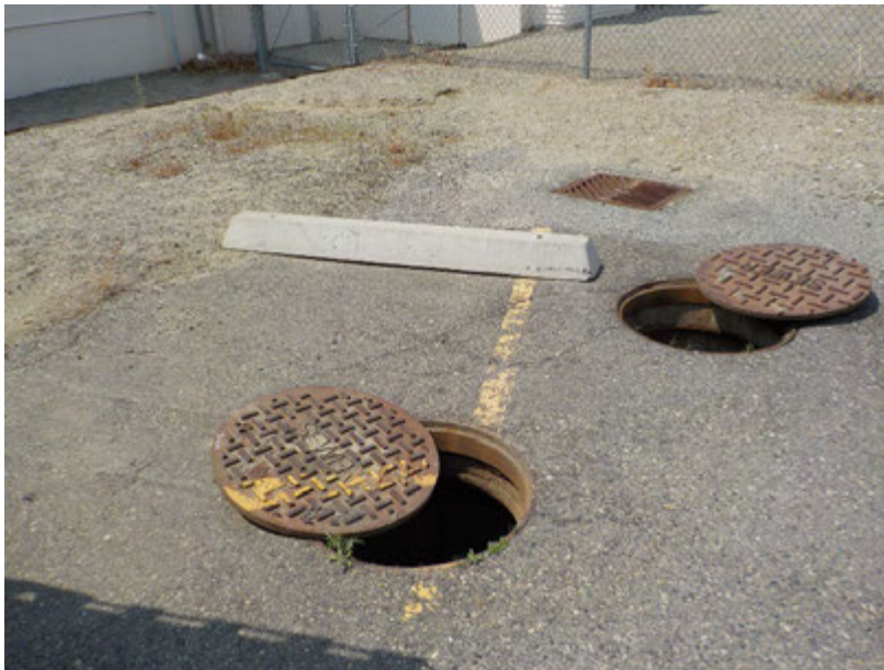
View of manholes at subject property septic system (northeast side of GA Terminal).
